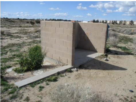
Concrete enclosure for a pad-mounted transformer on the subject property.
