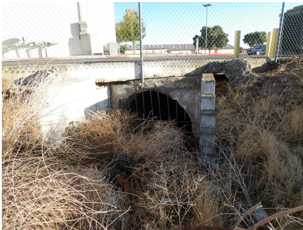
Photograph 6: Looking at the culvert located in the middle of the northern boundary marking the terminus of Drainage 1.
