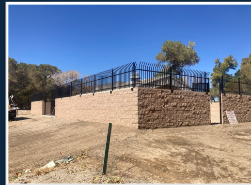
Stoddard Wells Lift Station
